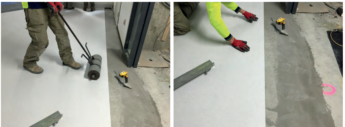
Before installing the floor coverings, the surfaces were levelled with ULTRAPLAN . The vinyl floor coverings were installed with ULTRABOND ECO V4 SP.
