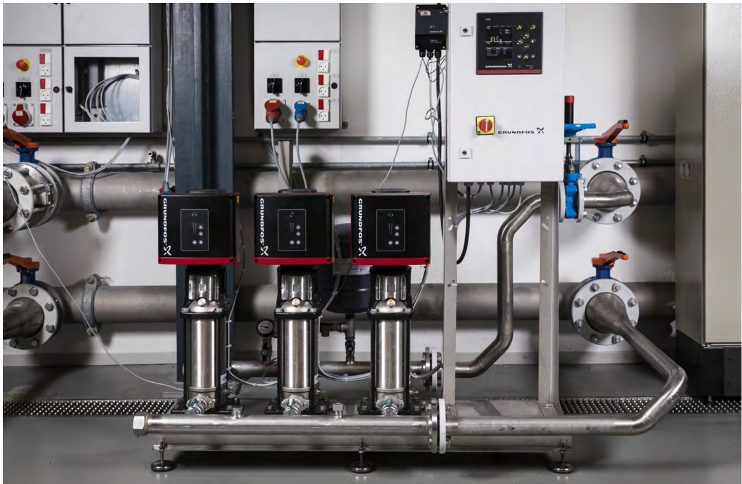
Installation of Grundfos Hydro MPC booster systems. Photo: © Grundfos Pumps Sdn Bhd
